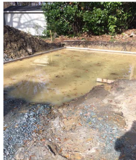
A neighbor's flooded construction zone.
